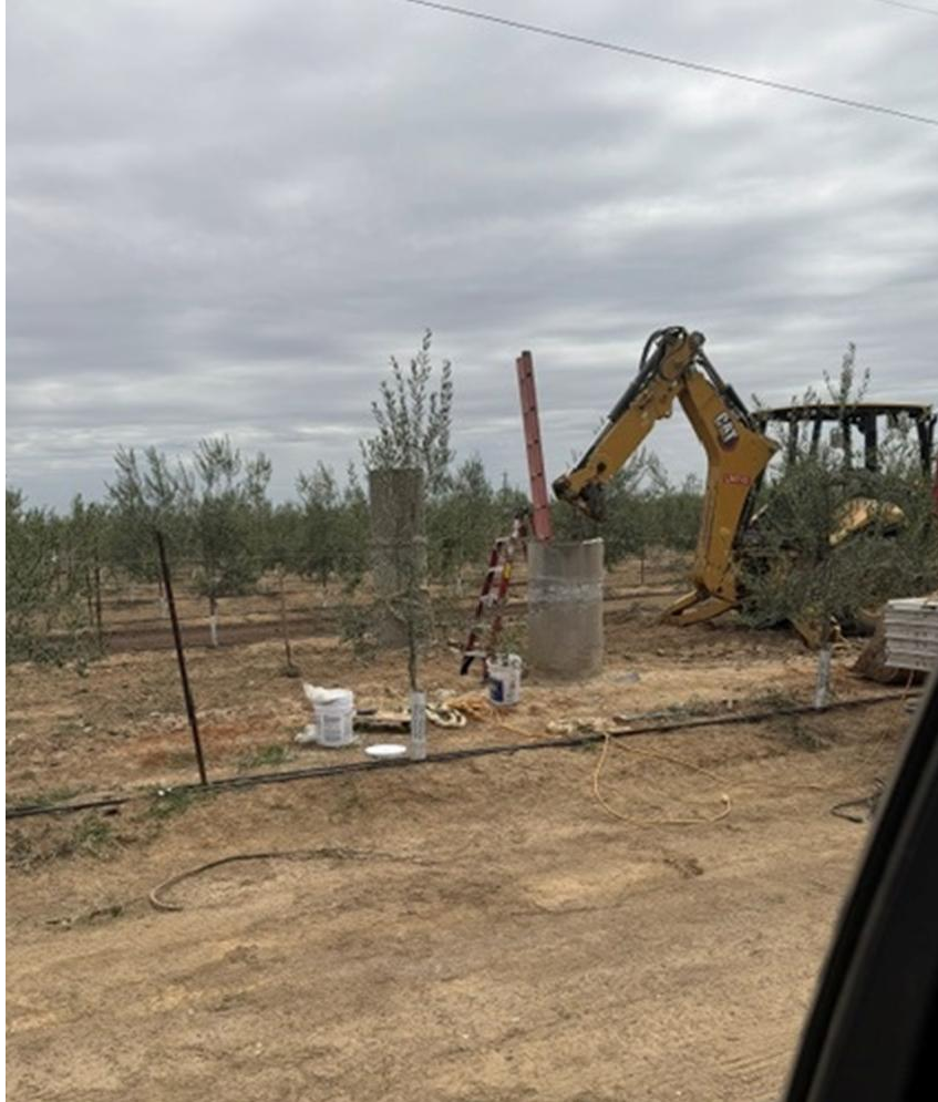
It's a pretty tight squeeze to repair the Tretheway Road section from inside
