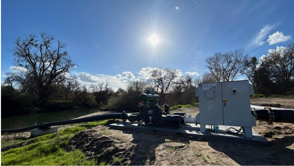
More power! The North pump station at full tilt while the fields can take more
