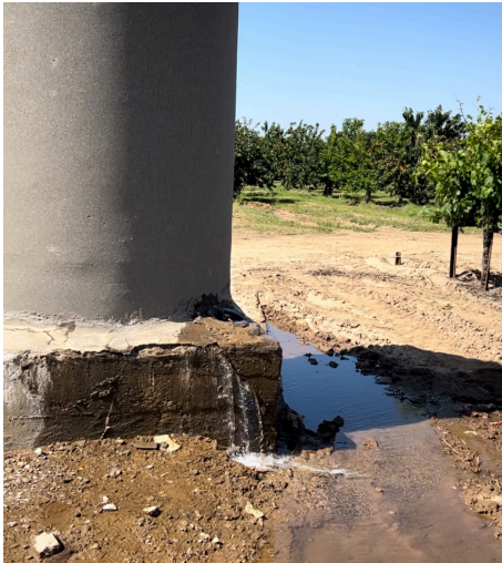
Phase 3 of the South System Improvement Project will fix leaks, including this stand pipe north of Kettleman Lane.
