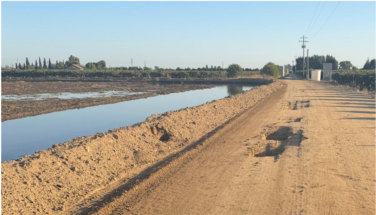
Compaction Failures developing in South System Phase 3 alignment
