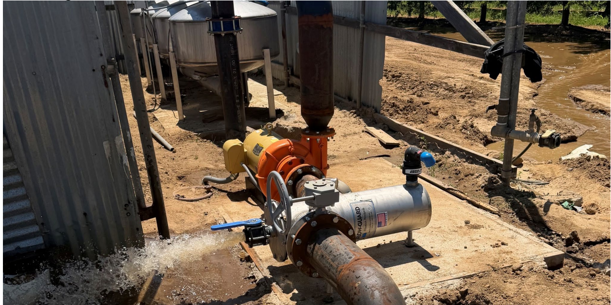
Surface Water Flows into North System Irrigation Lines
