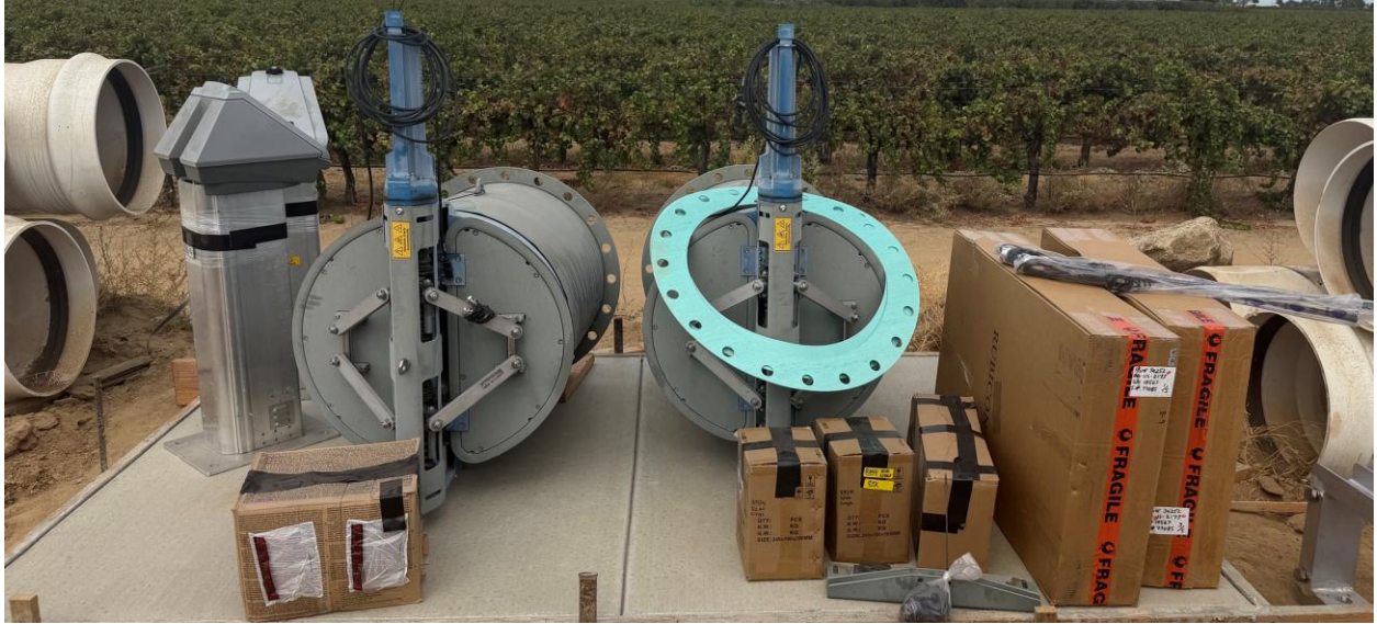
The New Rubicon automated valves and meters ready for install at Teck Basin
