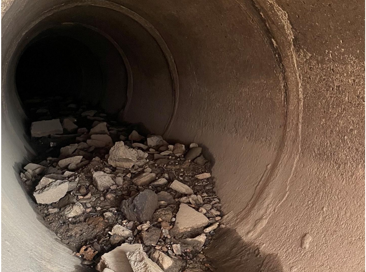
A few feet inside the Brandt Road Outfall to the East Ditch
