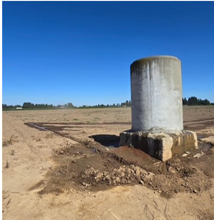
High Water Levels at Mettler Box feed a leak onto the Goehring Property
