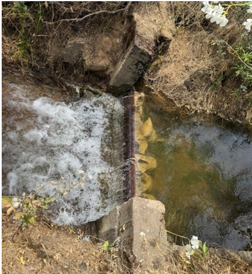
Water Pours over the East Ditch Dam at Lockeford Springs towards the main outfall into Bear
